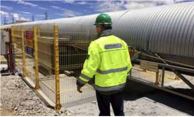
Figure 1. A CBGuard scanner with a safety fence in an overland conveyor.
